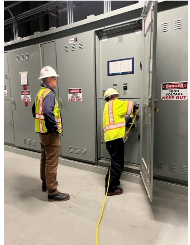
Salesforce Transit Center, 5-year electrical maintenance
